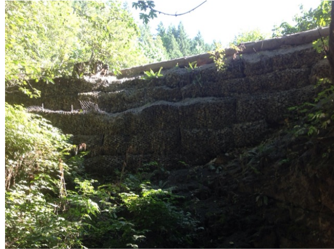
left upstream fill retention system
