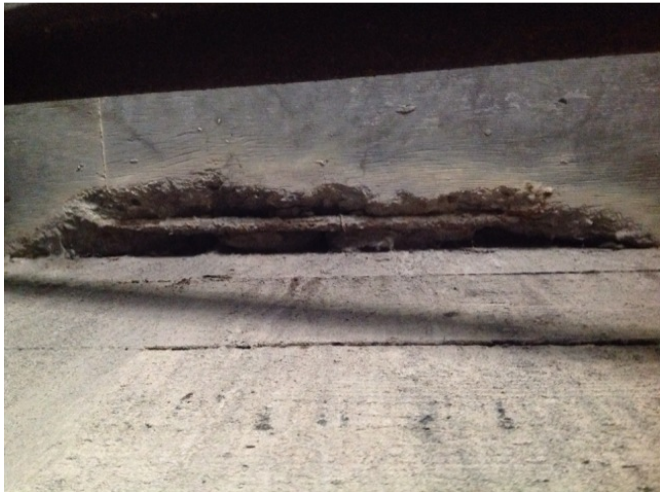
damage under panel 1
