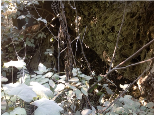
fill erosion left downstream approach under fill retention system
