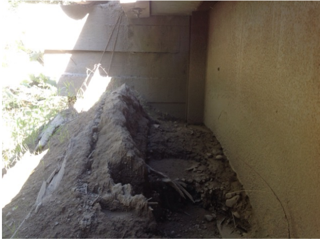
sediment covering bearing on left approach
